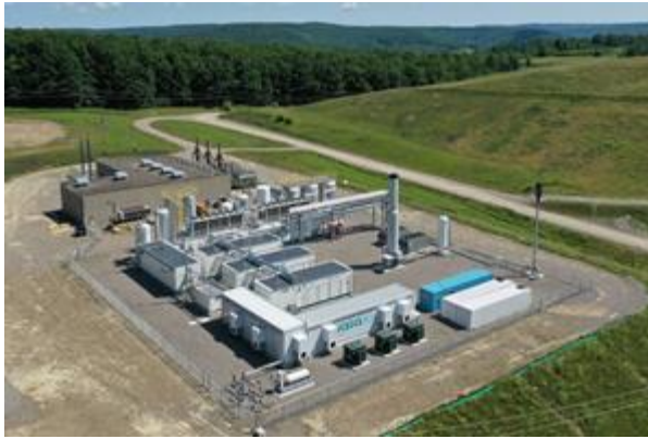
The Waga Energy Renewable Natural Gas Facility at Casella's Hyland Landfill in Angelica, NY
